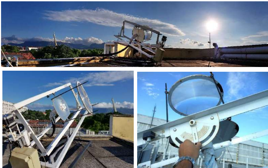
Figure 12. Upper: Solar tracker system installed on the roof of the Technology Center at the Universidade Federal do Rio de Janeiro. Bottom left: Details of the solar tracker, showing the stepper motor at center left, the microprocessor control box at bottom left, the Fresnel lens and the IR filter at the lens focus. Bottom right: Adjustment of the declination angle which allows the tracker to be directed to the sunrise direction.
