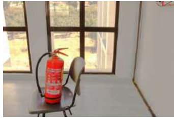
(b) Fire Extinguisher.
