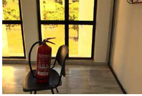
(b) Fire Extinguisher.
