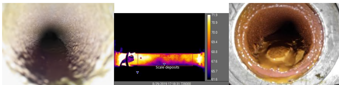
Figure 4.39: Scale deposits at pipeline bottom, indicated by lower temperature, the brown color indicated presence of Fe corrosion
