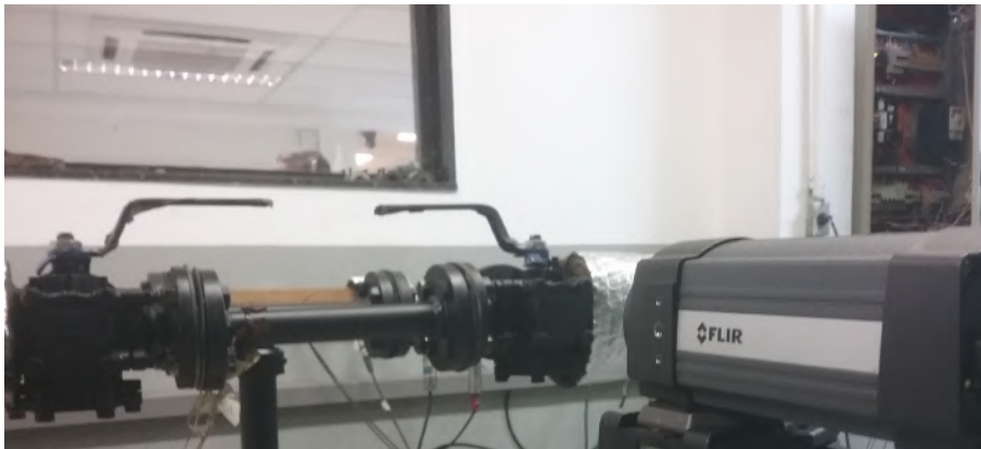
Figure 4.11: IR camera installed to detect pipe scaling
