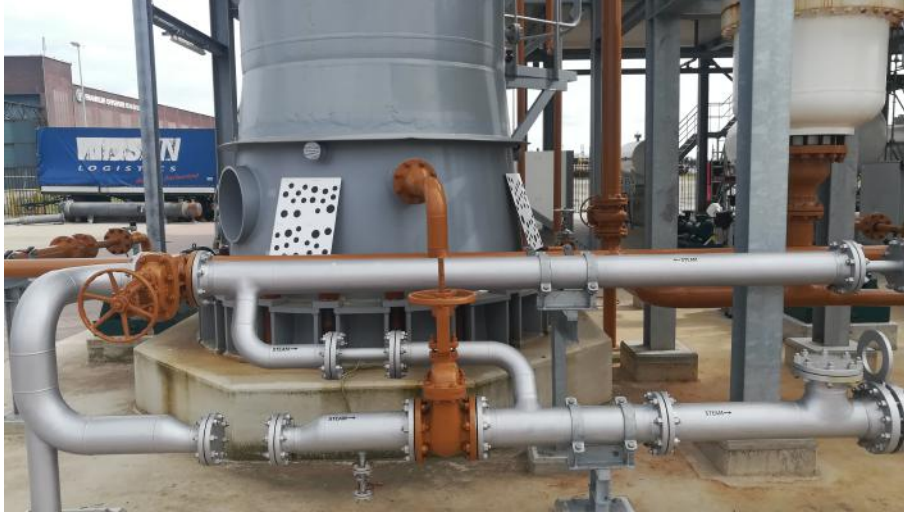
Figure 16: Refinery training plant flanges closeup.
