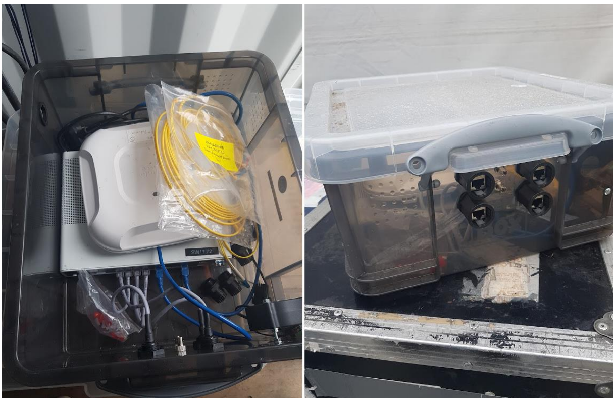
Figure 11 - Indoor 12-port switch and Access Point sealed and prepared for external usage. These boxes were mostly placed under bleachers and hidden in trees.
