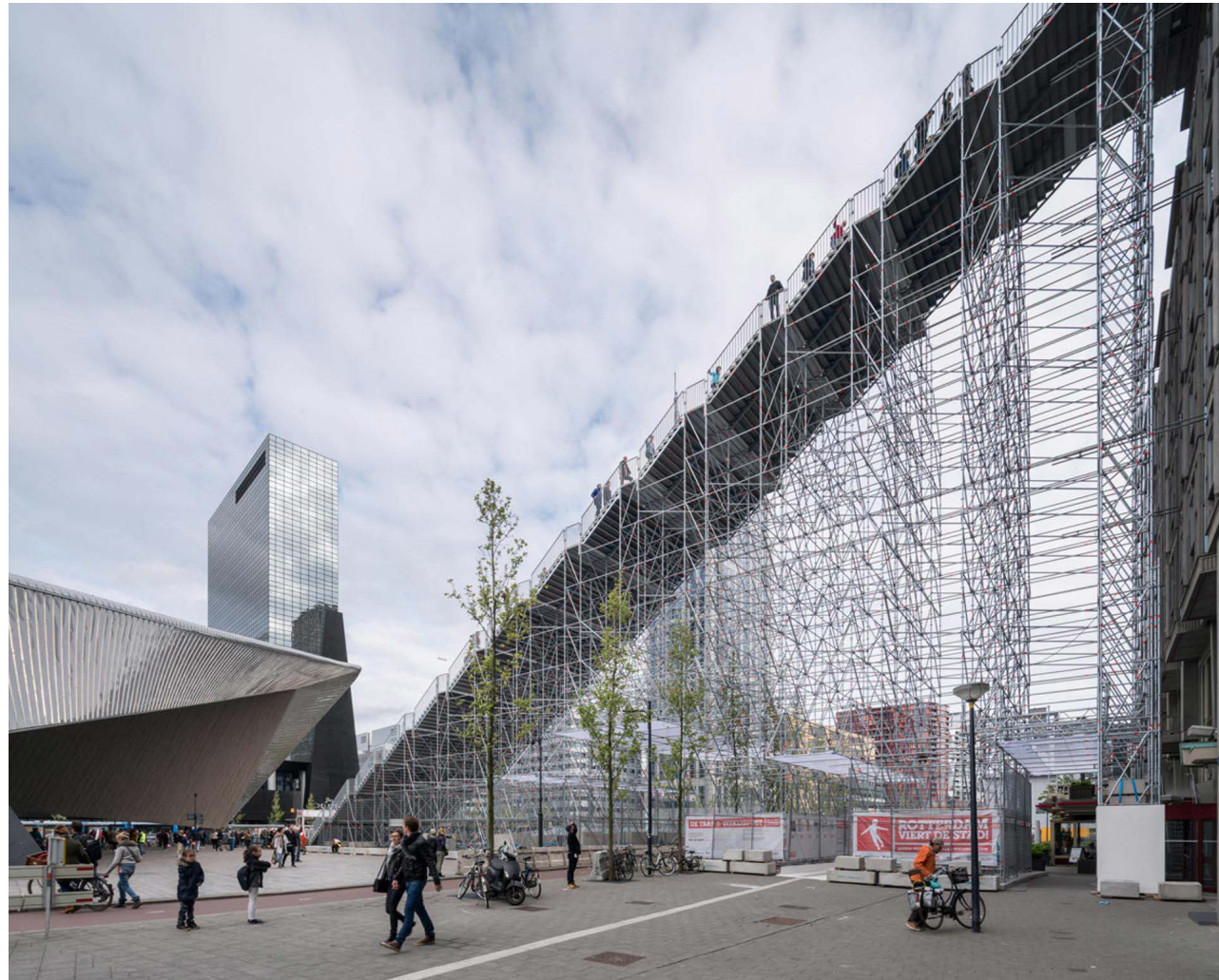
Stairs to Kriterion no evento 'Rotterdam celebrates the city!' - MVRDV (Fotos site MVRDV), (Rotterdam, 2016)
