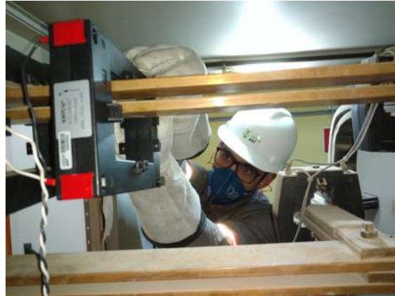
Figure 3.5: Installation of a current transformer by an electrical engineer on an appliance energy supply.
