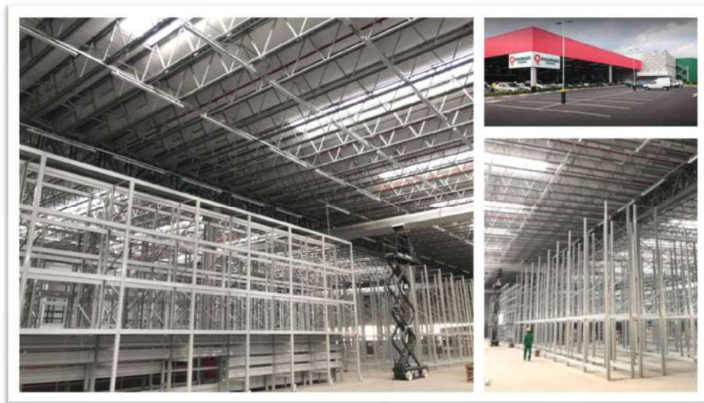
Figure 1.1. Roll-on roofing system from MARKO Sistemas Metalicos, consisted of cold-formed steel members, illustrated in the construction of Poupaki wholesaler, located in the city of Guarulhos, São Paulo, Brazil [4].
