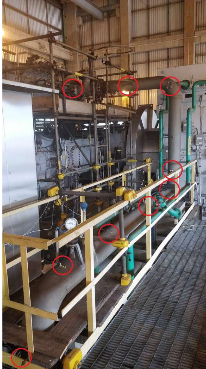
Figure 5.44: Second stage suction pipe with accelerometer installed highlighted with red circles.
