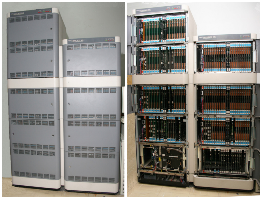
Figura 1 - Central NEC instalada no CT
