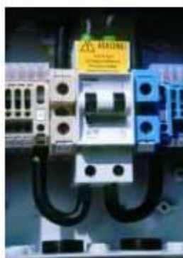
Figura 8 – Interruptor principal CC [2].
