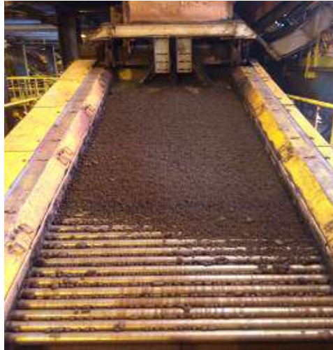
Figure 3.22. Roller screen in operation downstream from the disc pelletizer.
