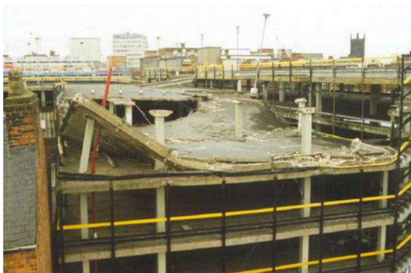
Figura 5.36 – Colapso parcial do Pipers Row Car Park (WOOD, 2003)
